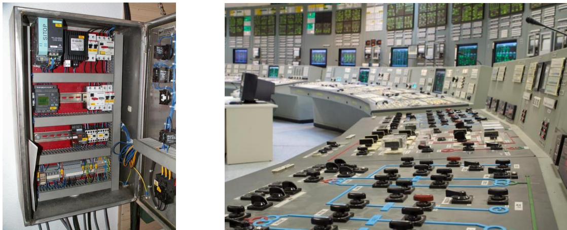
Figure 13 A control cabinet and a control room demonstrate the relationship between Faces and Visages.
